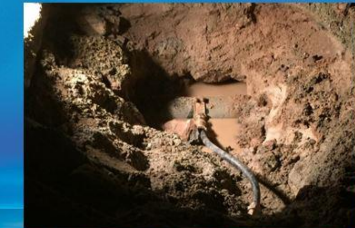
SANDSTONE CT SERVICE FAILURE 2018
