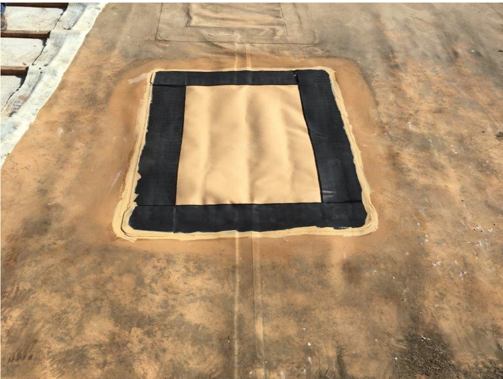
Figure 2. Photo showing typical completed patch with cover strips at sample extraction location. Note that repair and cover strips could not be completed with traditional adhesive methods. Cover strips used by CLI are Adhesive strips.
