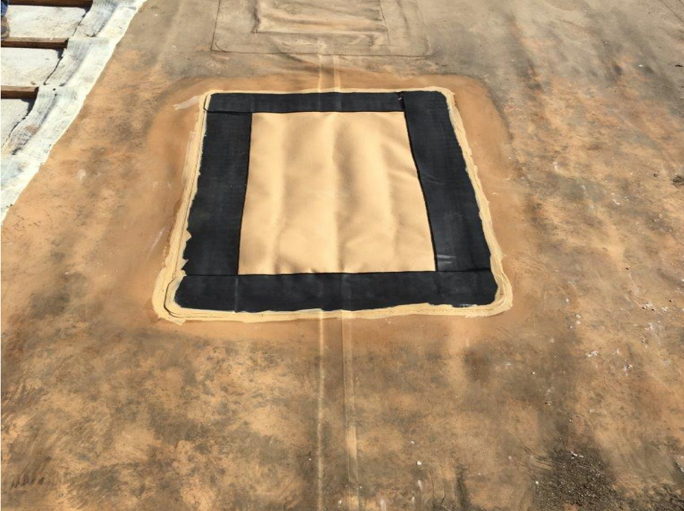
Figure 3. Photo showing typical completed patch with cover strips at sample extraction location.
