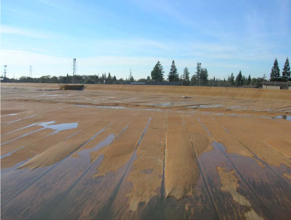
Figure 1. General View of the Hinkle Cover showing standing water, some discoloration, windblown silt/debris accumulation.
