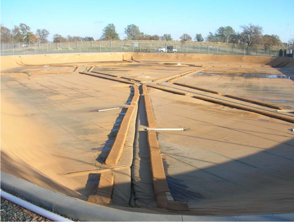
Figure 1. General View of the Kokila Cover showing irregular shape and Tensioned membrane design with sumps and floats.
