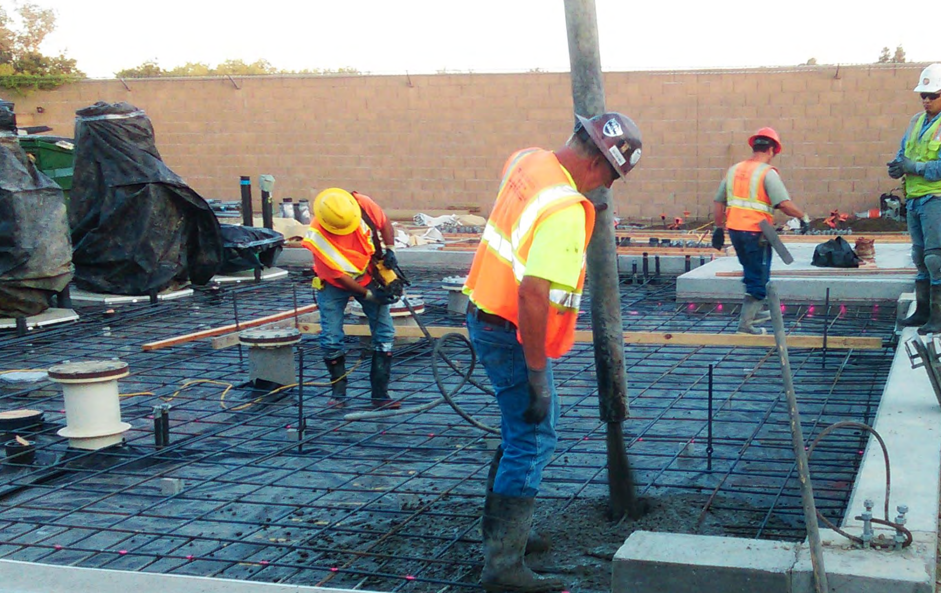
15, 6:09AM A slump sample was taken off the pump As the concrete pour started, Dana, with Paragon Ge
