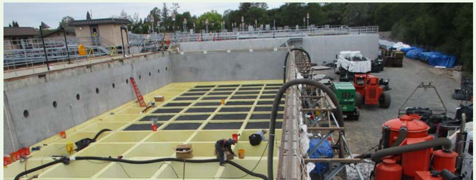
Rehabilitation underway on the two filter basins in our water filtration system at the Sidney N. Peterson Water Treatment Plant.
