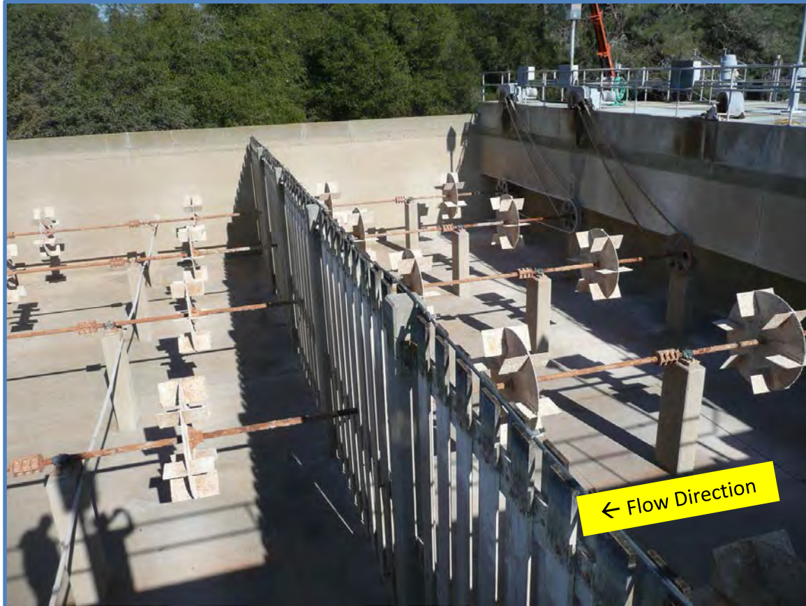
“BEFORE” – Turbine Type Flocculators
