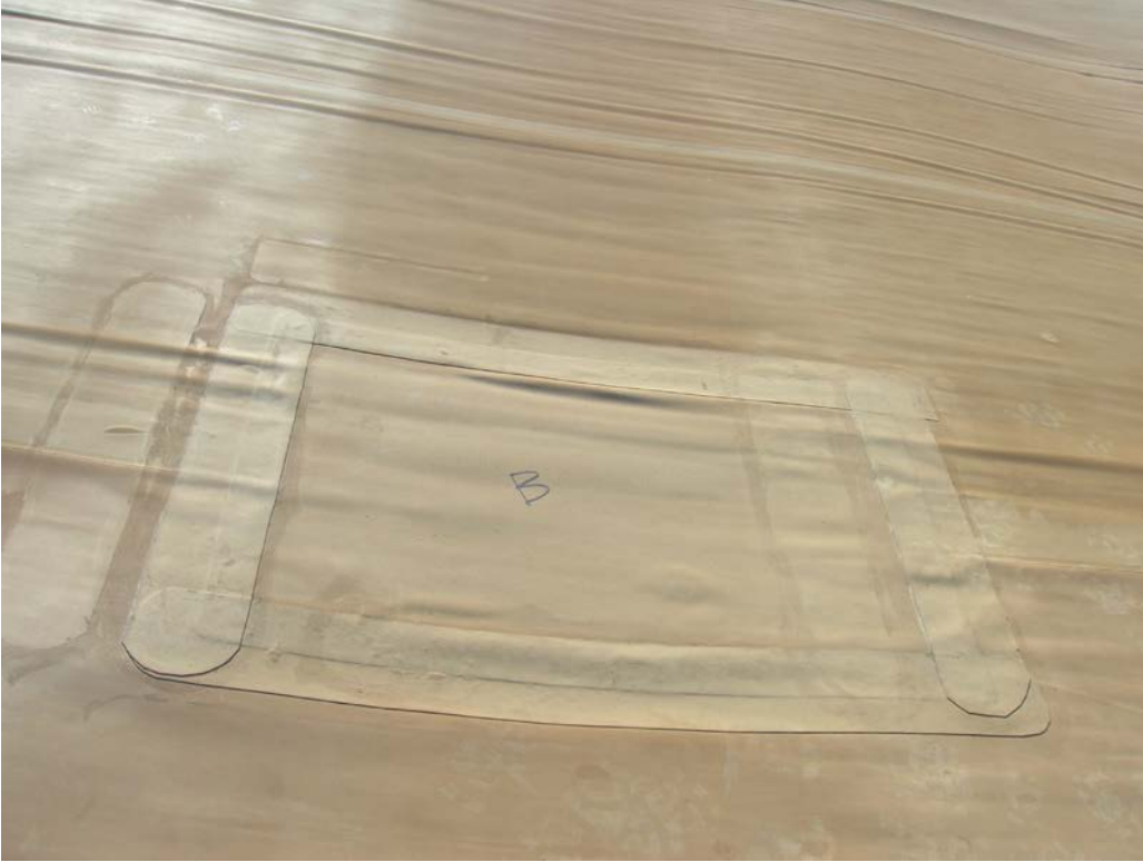
Figure 9. Photo showing original patch over 1999 sample extraction (B-1)
