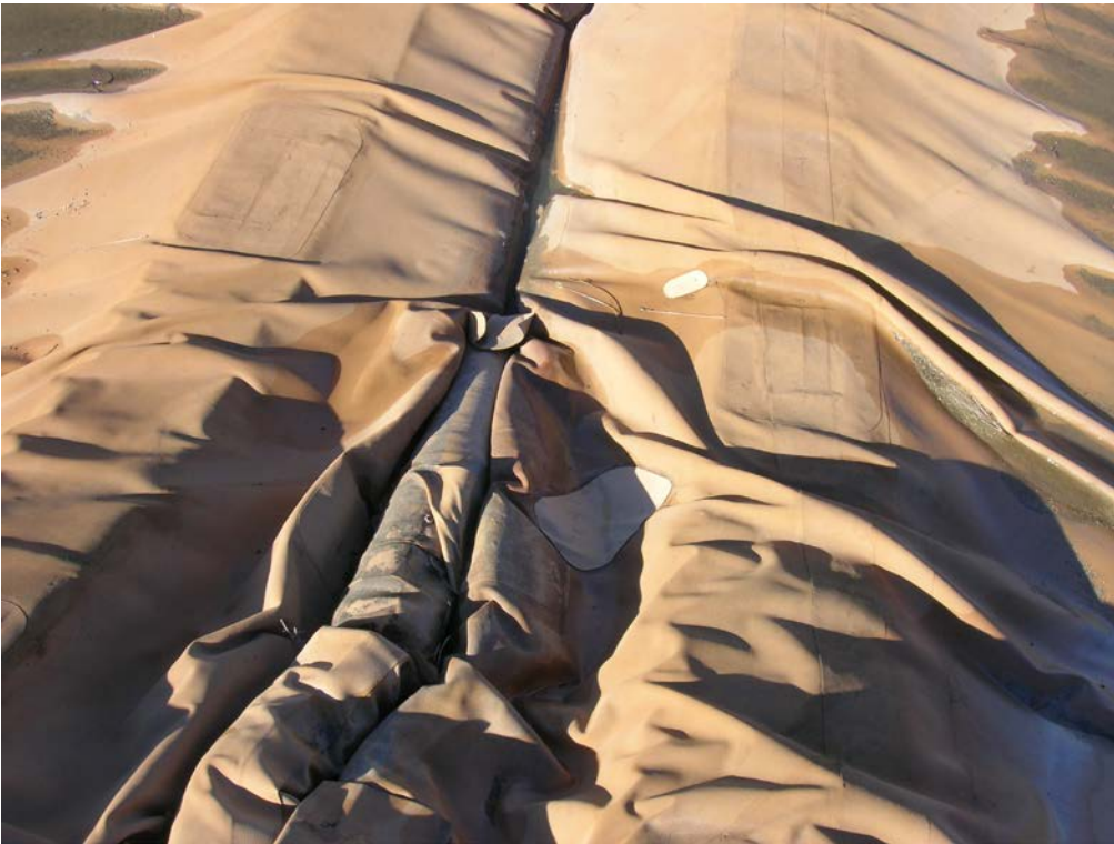
Figure 8. SE corner damage and repairs required due to high stress concentration.
