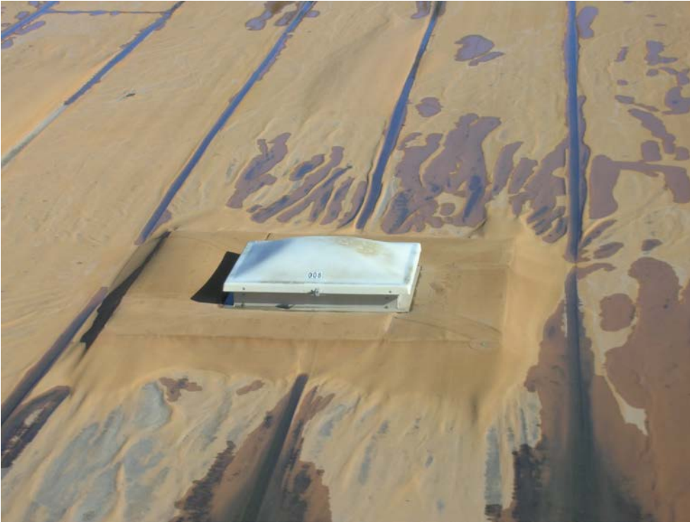
Figure 5. Photo showing one of 12 typical hatches on the Hinkle Cover with deteriorating fiberglass dome lids and supporting floatation system.
