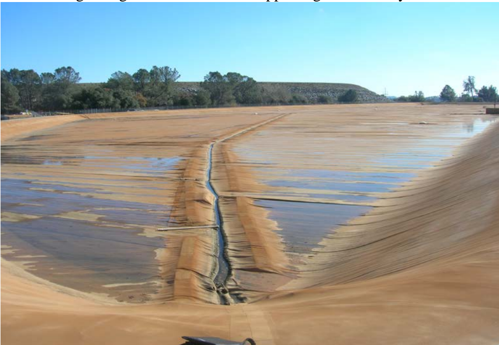
Figure 6. Photo at NW corner showing both standing water on cover and in sump line. Note that cover water is not getting to the sump and requires additional surface ballast or replacement of PVC tubes with 6 inch sand tubes.
