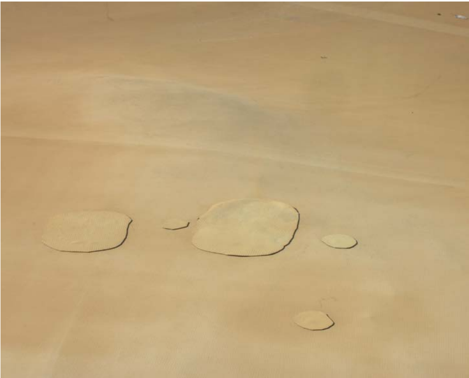
Figure 4. Photo showing poor quality adhesion and irregular patches.
