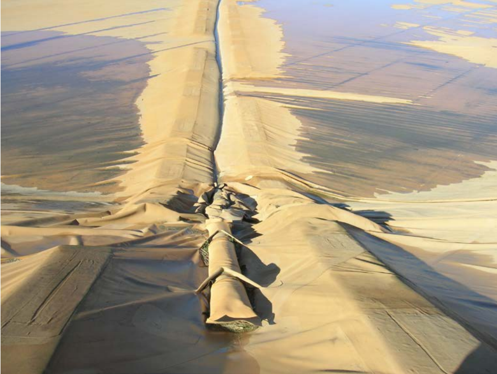
Figure 7. Photo showing the distortion, misalignment and damage at the SE Corner.
