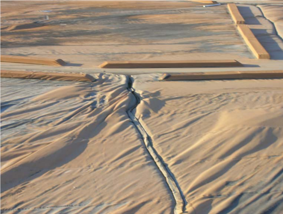
Figure 11. Excessive distortion and wrinkling of the cover which is impeding the flow of rainwater to the sump as illustrated by the dark coloration to the left of the wrinkle.
