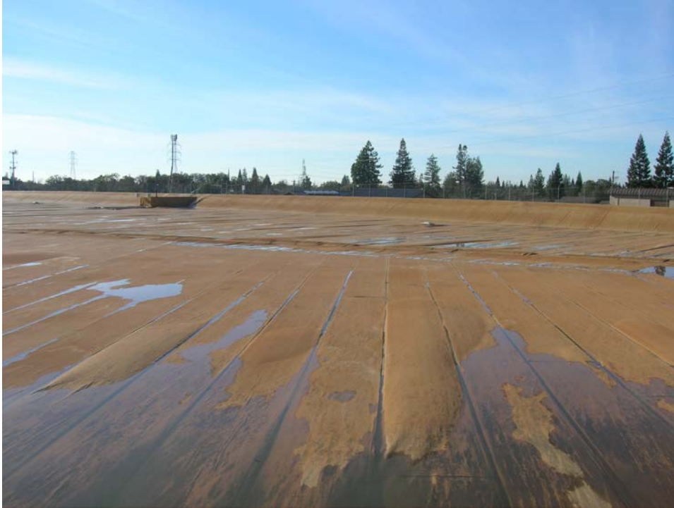
Figure 1. General View of the Hinkle Cover showing standing water, some Discoloration, windblown silt/debris accumulation and minor air entrapment
