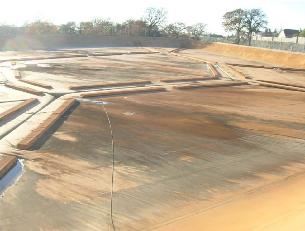
Figure 12. SE quadrant section showing very dark discoloration (due to standing water) as well as windblown silt and debris.
