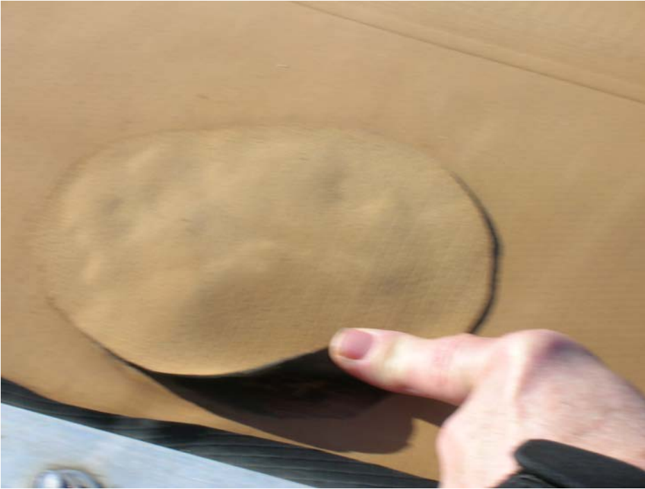
Figure 3. Photo showing poorly adhered patch with blistering.
