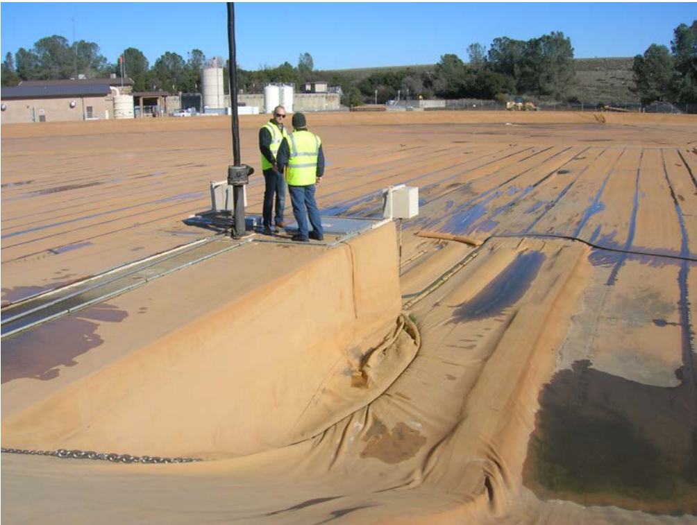
Figure 10. Outlet Structure with re-designed and functioning float/ballast system.
