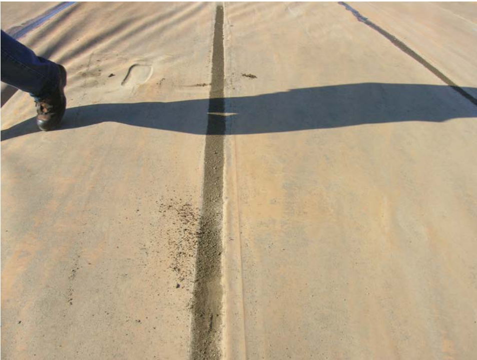
Figure 4. Typical factory seam over water with accumulated windblown dirt and debris which should be removed during the next cleaning operation.
