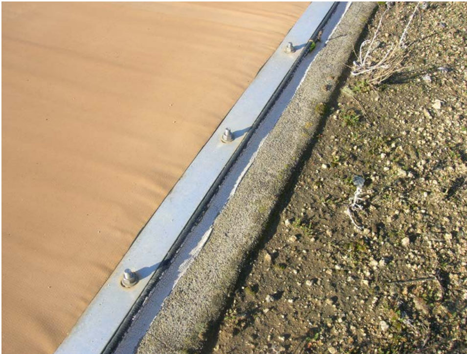
Figure 2. Photo showing typical condition of the perimeter attachment.
