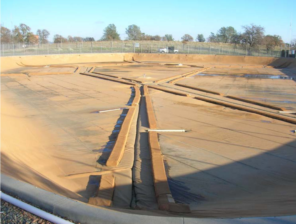
Figure 1. General View of the Kokila Cover showing minor surface water, discoloration, windblown silt/debris as well as surface ballast tubes. Note surface bonded floats
